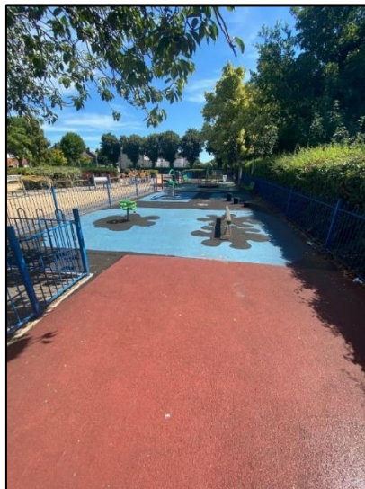
Poor quality play surfacing
